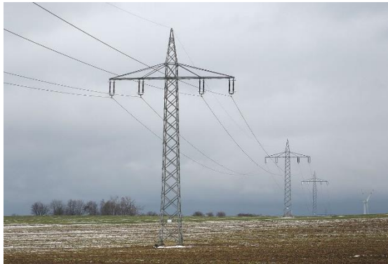
Figure 2.1: 110 kV distribution line
