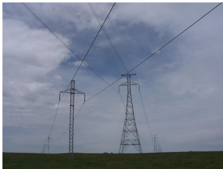
Figure 2.3: Transmission tower for a HVDC line
